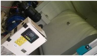
- 7 gensets 22 kVA installed in containers
